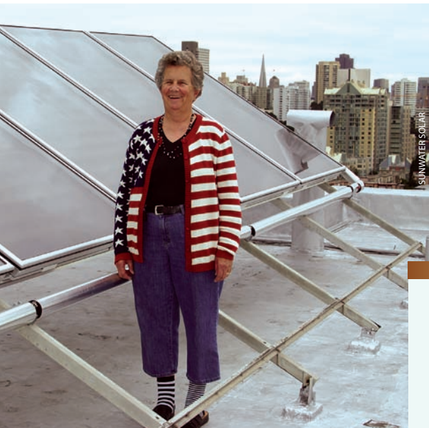
Author Linda Erkelens shows off some of the 14 Schüco collectors that provide 1,277 therms per year at her 21-unit apartment building.
