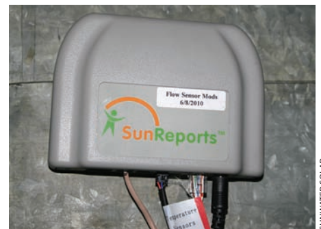
A SunReports sensor box collects data and sends it out to a web portal for remote monitoring of temperatures and pump status from anywhere with internet access.
